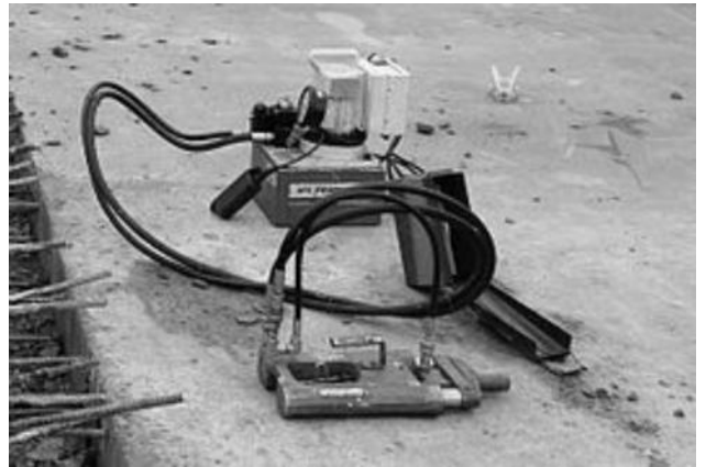
Hydraulic jack for tension cables
