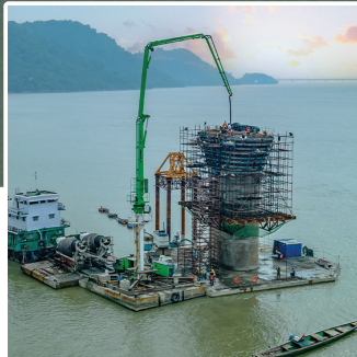
SEPARATE PLACING BOOM
